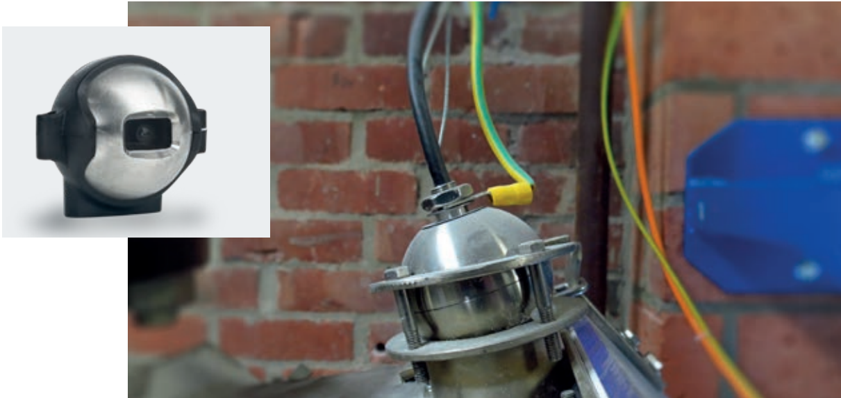
Inspection window monitoring at the boiler using the EC-710 camera
