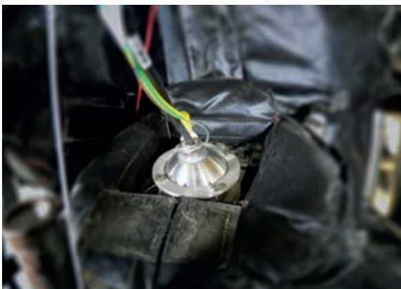
EC-710 at the front of inlet enclosure
